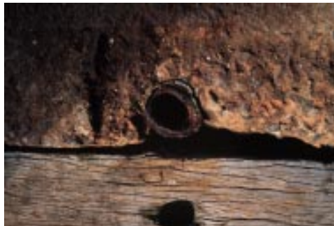
Metal blow hole in Kirribilli Wharf
